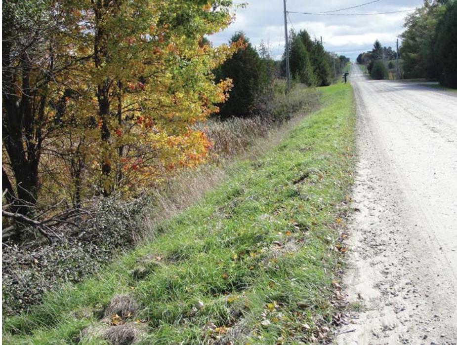
The shoulder drops off well before it measures 1 metre in width.
