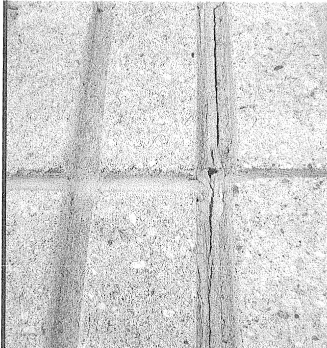
Cracked joint sealant needs replacing.
