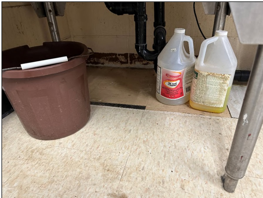
Photograph 3: View of six tiles of asbestos-containing 12" beige vinyl floor tiles with white and black streaks (VFT-B) under the sink in the Concession Stank (Location 123), assigned a Priority 2 .
