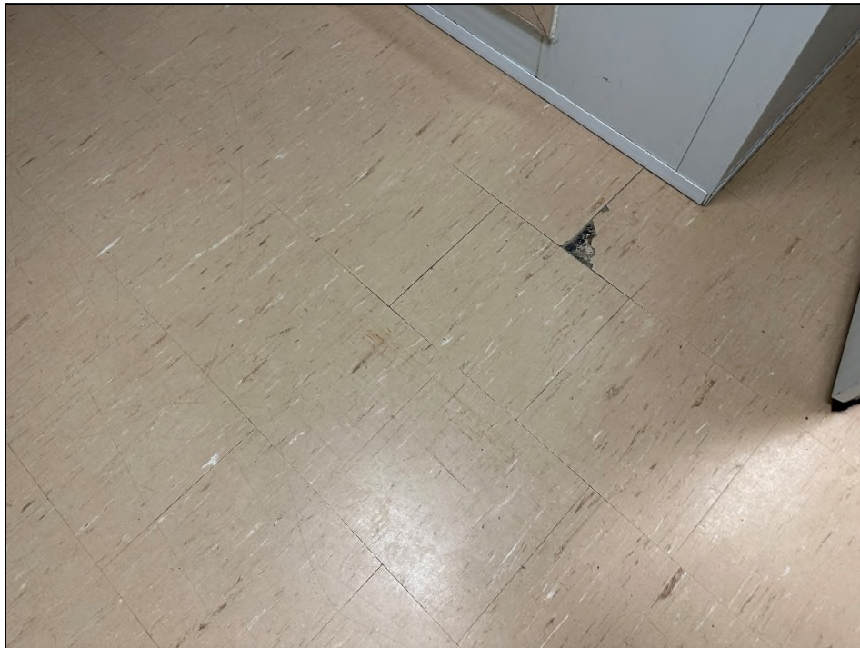
Photograph 1: View of asbestos-containing 12" beige vinyl floor tiles with white and black streaks (VFT-B) in the Bar/Freezer Room (Location 105), assigned a Priority 2 .
