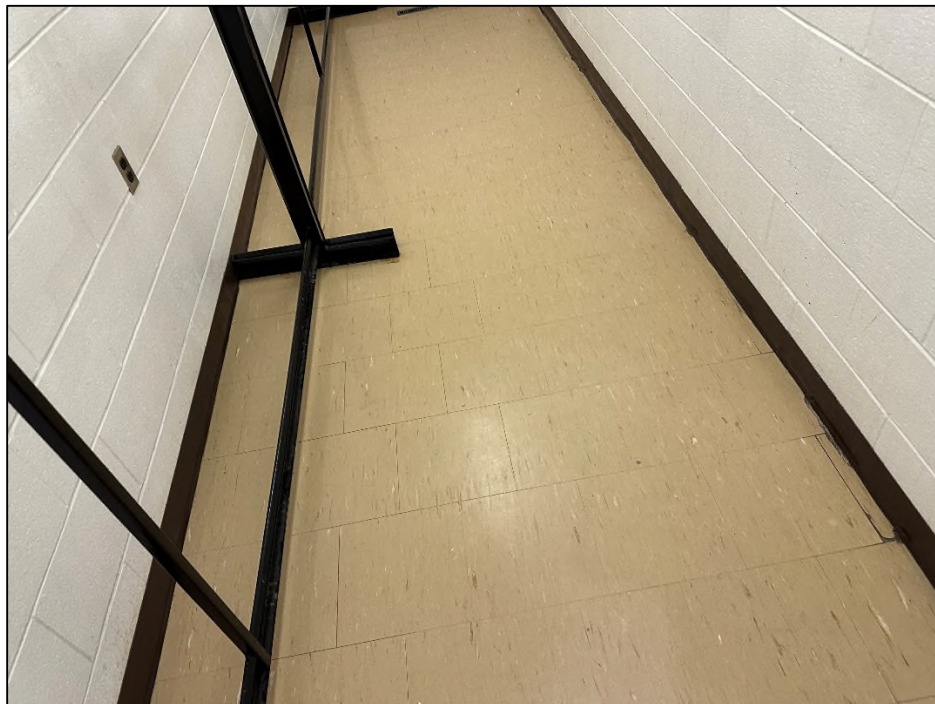
Photograph 2: View of asbestos-containing 12" beige vinyl floor tiles with white and black streaks (VFT-B) in the Coat Room (Location 107), assigned a Priority 2 .
